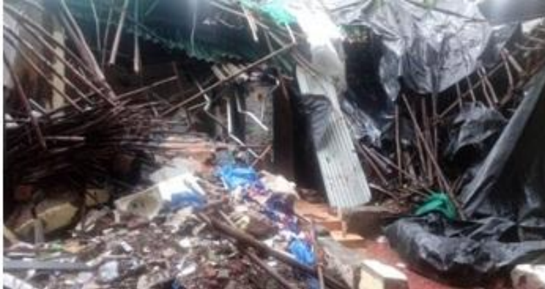
Closer View of the Demolished Structure from main entrance
